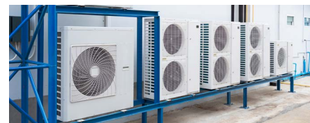
CENTRAL HEAT PUMP PLANT
