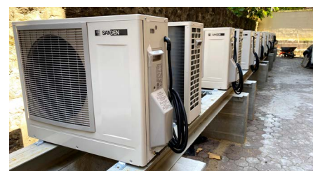
CENTRAL SPLIT HPWH PLANT
