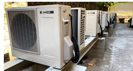
CENTRAL SPLIT HPWH PLANT
