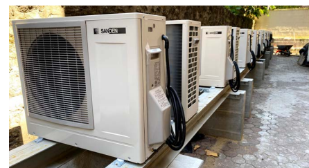
CENTRAL SPLIT HPWH PLANT
