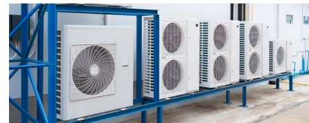
CENTRAL HEAT PUMP PLANT
